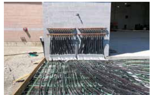
Manifolds keep the snow melt and radiant systems running smoothly.
