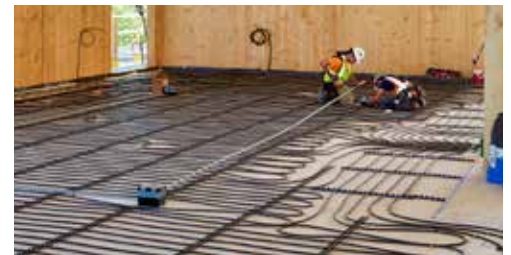
Both buildings are comfortable thanks to radiant heating and cooling products.
