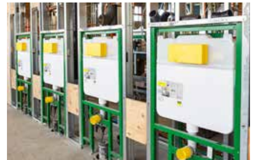
Viega Flushing System Technology is featured in the seminar center and headquarters buildings.
