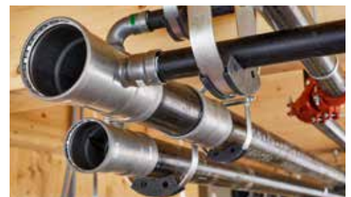
MegaPress connects the fire sprinkler system and MegaPressG fittings were used on the natural gas lines.
