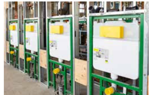
Viega Flushing System Technology is featured in the seminar center and headquarters buildings.
