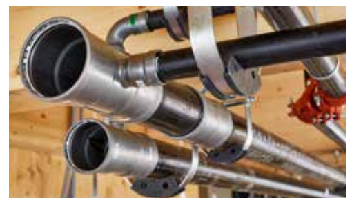
MegaPress connects the fire sprinkler system and MegaPressG fittings were used on the natural gas lines.
